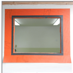
11. Immediately spread the applied material with a putty knife creating a 1" border around the rough opening.
