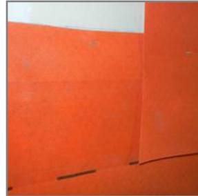
3. Line up the bottom of the upper course of material with the dotted line, creating a 6" overlap.
