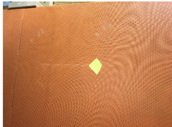
Membrane abrasion and hole, prior to repair with VAPROBOND.
